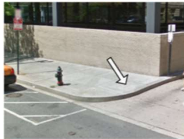
Missing Curb Ramps
